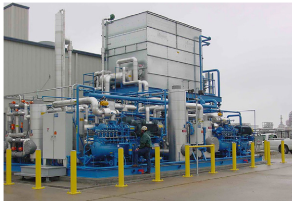
CO2 plant alongside raw gas source.
